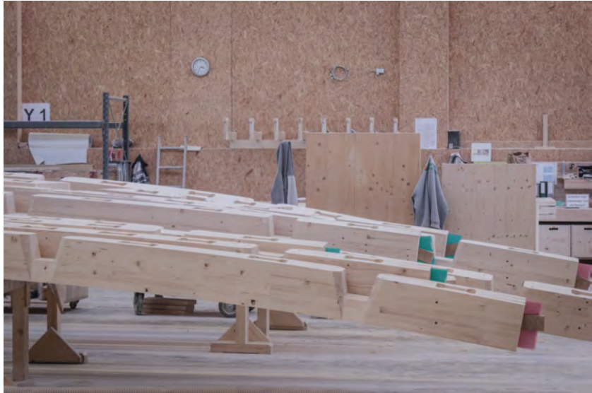
Fig. 5.15: Crossing lap joints require the removal of a large portion of the glulam cross-section.
