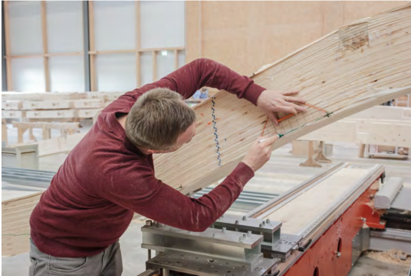
(a) Tracing the production data on the material to measure the alignment deviation.
